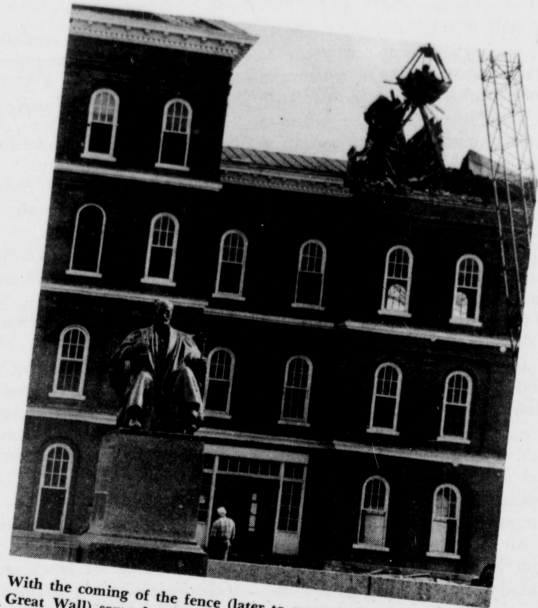
Returning students found a giant fence built around the construction site of the new Administration-Classroom Complex. A student takes advantage of the vantage point to watch workmen . . . but the fence was to be only the beginning . . .
