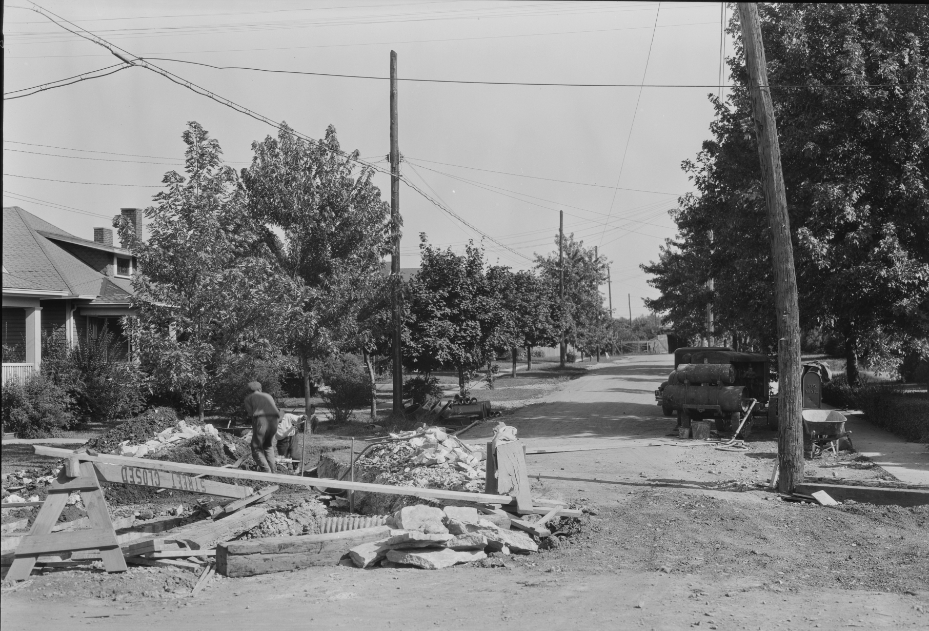
CITY OF LEXINGTON Richmond & Aurora Ave Sta. 54+75 East Contract No. 3 CONNELLY BROS 9-6-34
