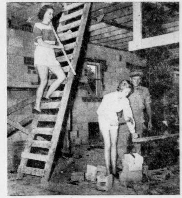
Chi Omega's Spencer McClure (on ladder) and Liz Ross, helped out at the new Chi O house which is going up on Rose Street. Workman Carl Jones seems a little concerned about Liz's ability with a hammer.
