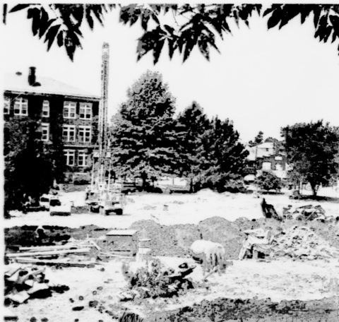
Construction is now under way on the new College of Commerce Building, near the main entrance to the University on South Limestone Street. The new building will replace White Hall, which has housed the College of Commerce for more than 40 years.
