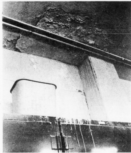
Leaks like this are common in Funkhouser. A pump keeps the basement dry during spring rains.
