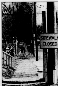
PHOTOS BY JAMES CRISP/Kannel staff GRIDLOCKED Construction workers keep busy on Columbia Avenue. Library construction increases traffic (top left). Sidewalks are closed at Rose and Columbia (above). A hole next to the Delta Gamma house will contain a manhole (right).
