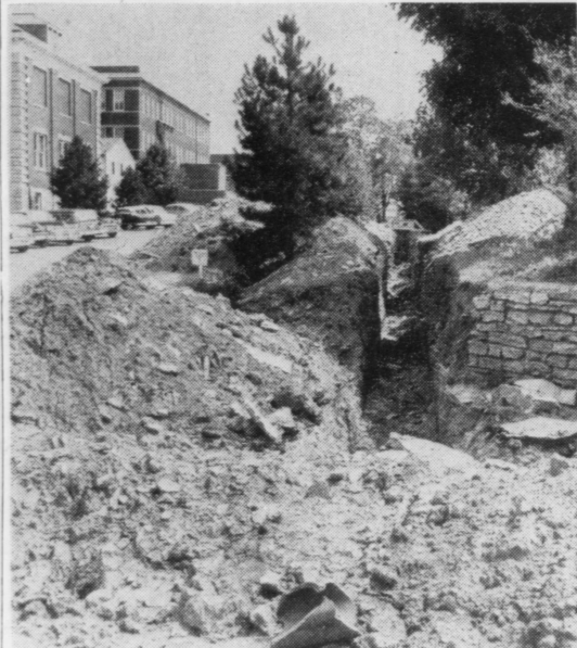
THE DITCH running around and through the tennis courts is not to keep people from playing tennis. It is to be the steamline for the new boys dorm on Rose Street.
