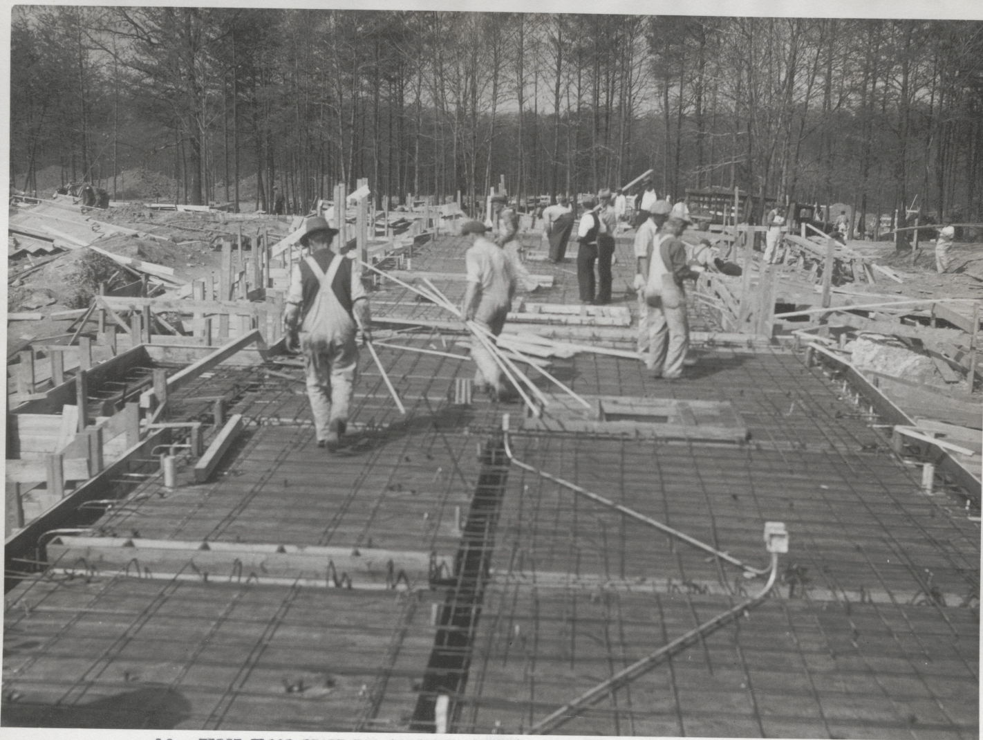
12 - FIRST FLOOR READY FOR CONCRETE, REINFORCING STEEL, PLUMBING AND HEATING SLEEVES, AND ELECTRIC CONDUIT SET
