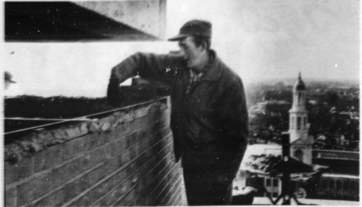
of the campus. Still the construction goes on. The interior of the building is the focus of attention now. At left, huge pieces of equipment are being used for the completion of the top floors of the building. The target date for the opening of at least three of the classroom
