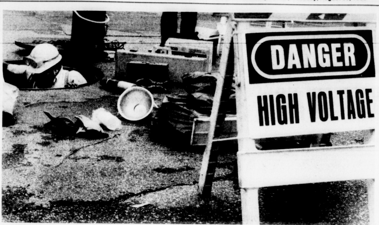
UNDER COVER: A UK Physical Plant Division employee crawls out of a manhole by the Chemistry/Physics building, located on central campus. The workers were working to replace an underground high voltage line.
