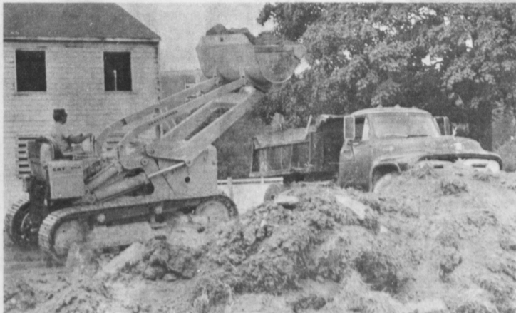
Men are now busy on the excavation work for the new law building.
