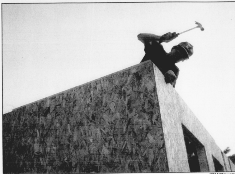
Jeff Herrin, president of UK's Habitat for Humanity chapter, helped build a house at 425 Hawkins Ave. in downtown Lexington. Construction began yesterday morning and is expected to be completed this week.
