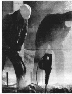
David Floyd (left) and Johnny Poynter are hard at work on UK's new Plant Science Building.
