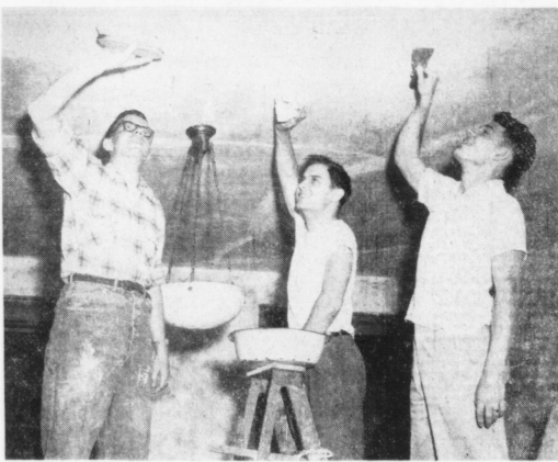
WESLEY WORKERS —Three members of Wesley Foundation pitch in to help with the remodeling of their Maxwell Street center. They are, l. to r., Edmund Young, Don Mosley, and Leroy Bondurant.
