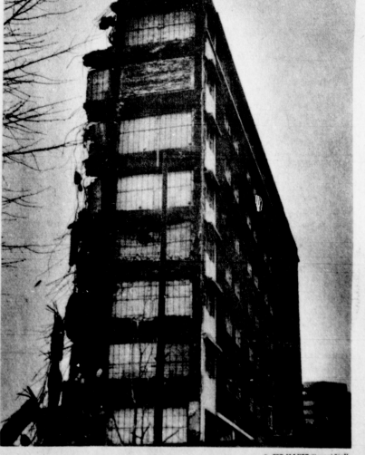
The Phoenix Hotel located on Main Street in its final stages of demolition.
