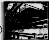
All steam, water and compressed air pipe-lines in the Goodyear plant are Crane materials.
