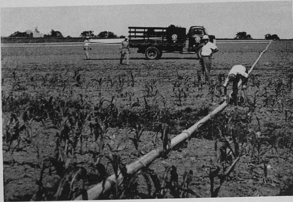
Fig. 5.— Portable pipe lines with quick couplers are laid on top of the ground.
