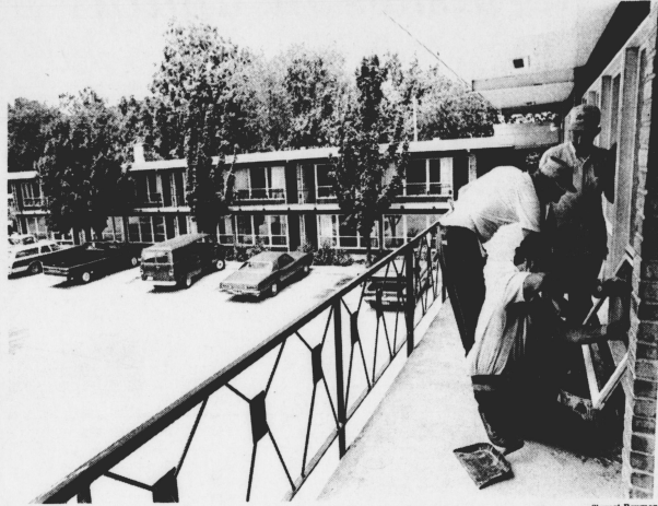
Workers are now busy cleaning and repainting the Holly Tree Manor apartments that UK purchased. The complex, composed of efficiencies and one-bedroom apartments, will be ready for occupancy by graduate
