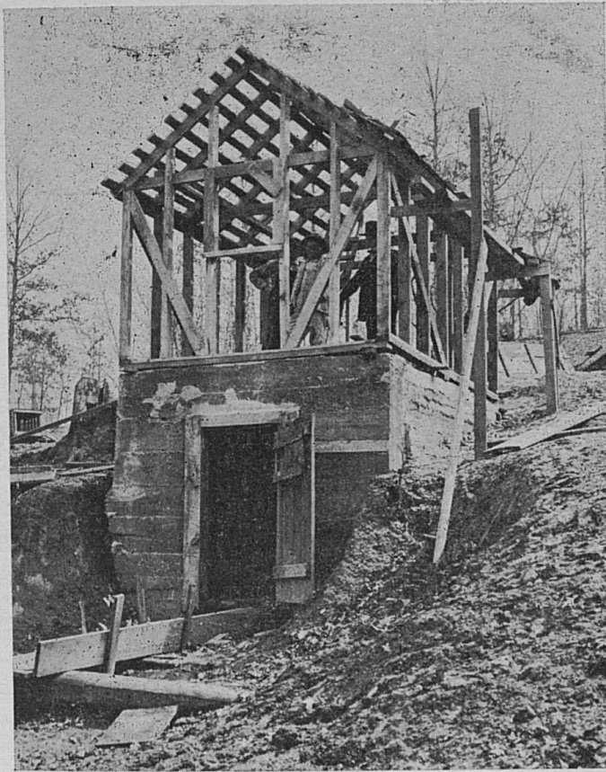
Fig. 15. A Concrete Hillside Potato Cellar; the Second Story for Storing Sweetpotatoes.
