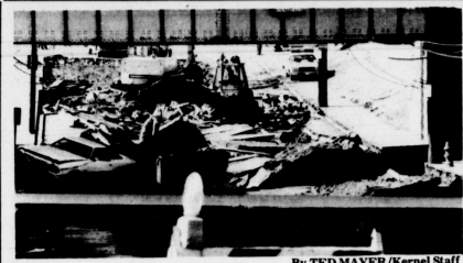
This Louisville street was torn up by a violent gas explosion Friday morning.
