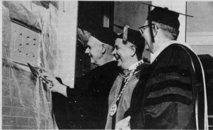
Smoothing cement around the cornerstone at the new Somerset Community College are Louis Ware, left, dedicatory speaker, and Dr. John W. Oswald. Dr. Lawrence Davenport, director of the UK branch, looks on.
