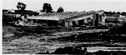
The new football stadium is taking shape after several weeks of construction. The stadium, located on Copper Drive, should be completed in time for the first game next fall. (Kernel photo by Skip Garrison)
