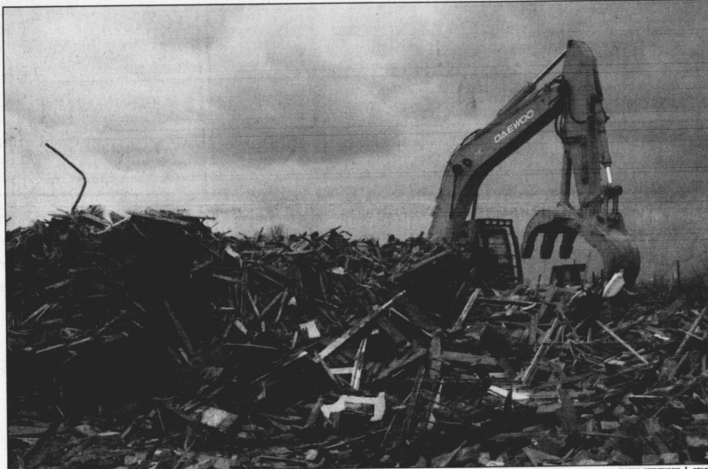
Workers move rubble tearing down the buildings at the corner of Limestone Street and Transcript Avenue yesterday as part of UK's hospital expansion.
