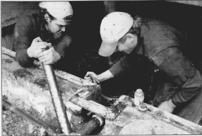
Workers Scott Bowman and Jimmie Shackelford from DC Elevator company replaced a broken hydraulic pipe yesterday at the UK Stores Building on Scott Street.
