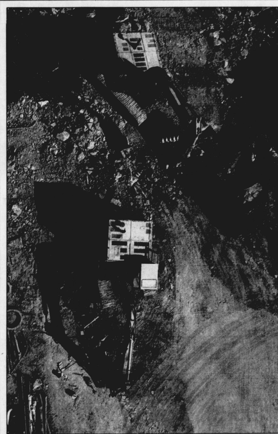
SHAKE, RATTLE AND ROLL: While construction on a new engineering likely will continue through the school year, blasting that accompanies it probably will subside after March.
