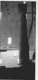
The second floor Public Room will be used for press conferences and other gatherings. The pillars were one of the few parts of the building that survived the May 2001 fire. JONATHAN PALMER | STAFF
