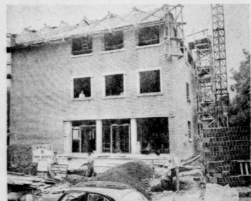
UK'S BUILDING CONTINUES as workmen approach the final stages of outside work on the new Mines and Minerals building.
