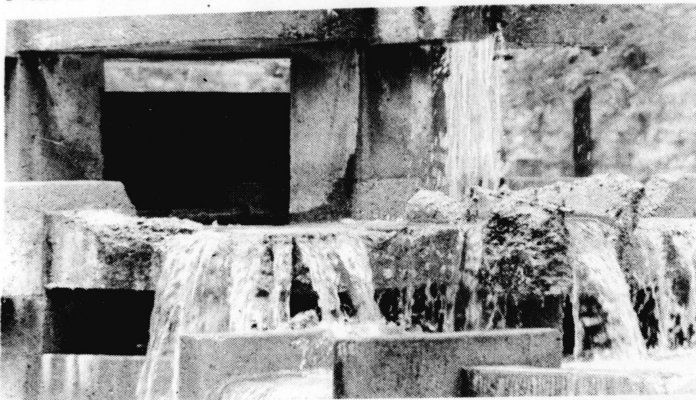
The 10-year-old fountain in the Patterson Office Tower plaza is beginning to show its age as it deteriorates piece by piece. The fountain, which was built in 1969 with the Office Tower, will soon be replaced if acceptable bids are received from contractors.
