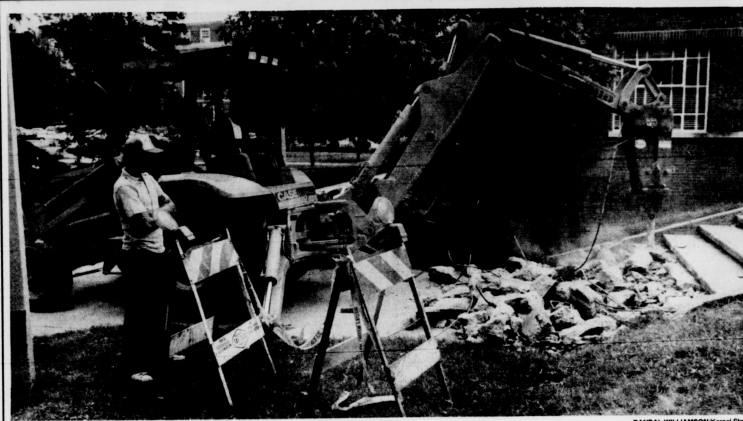
Two employees of Peipe Works Construction Co. hoist a set of steps by the UK law building yesterday afternoon. The company was contracted to replace several sets of deteriorating steps on the University campus.
