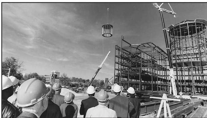
Bystanders watch as the six ton cupola of the William T. Young Library is raised onto the building during construction in the Fall of 1995.
