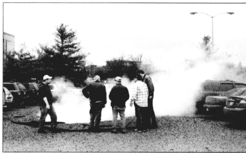
Physical Plant workers gather around the hole left by a steam pipe that ruptured yesterday in the Kentucky Tobacco Research and Development Center parking lot.
