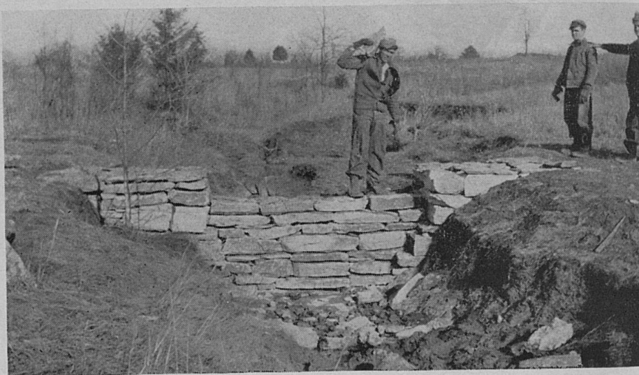
Stone dams, with black locust trees planted on the sloped gully banks in the rear, may be used to check soil out-wash while the trees' roots are getting firmly established.
