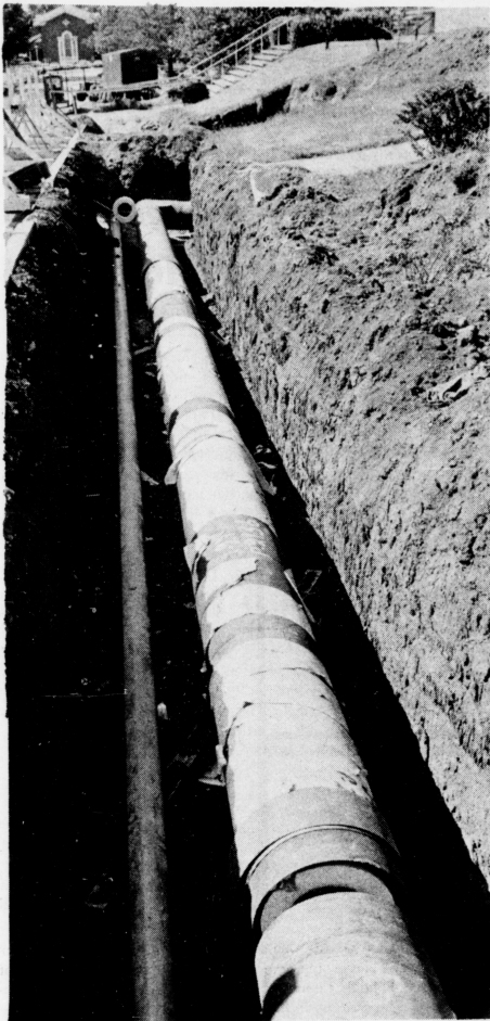
Don't get all steamed up about open trenches like these scattered across campus. Workmen are trying hard to complete this network of heating pipelines before winter comes. The important thing is not to fall and break your leg.
