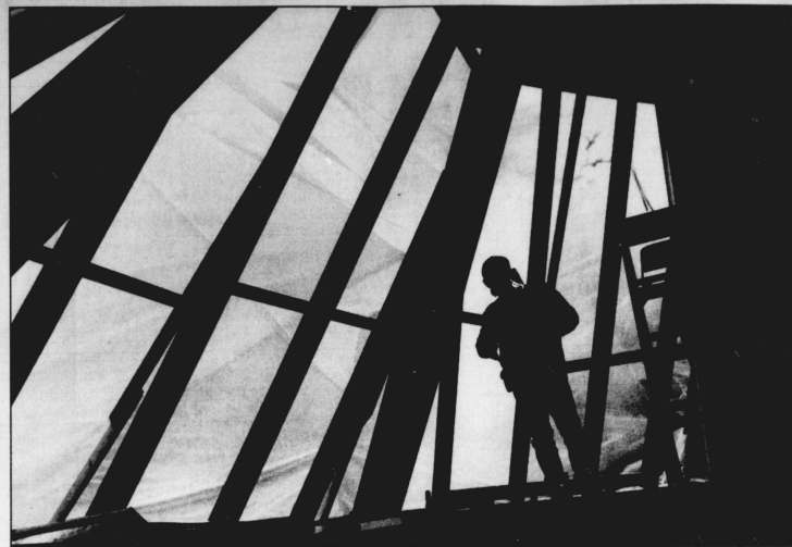
Rodney Clephane works on a new skylight on the roof of the Ezra D. Gillis Building.
