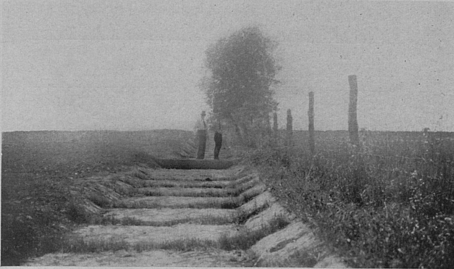
Fig. 11. A low concrete dam used to reduce the grade in an outlet channel.
