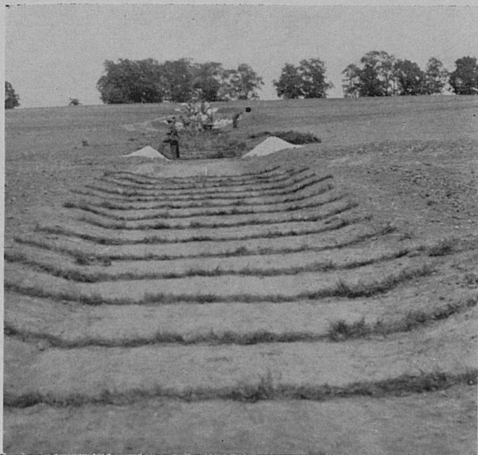
Fig. 7. Sod strips used to check erosion in an outlet channel while sod is being established from seed.
