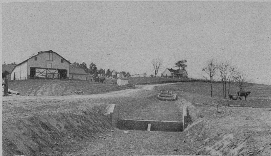
Fig. 9. A terrace outlet protected from erosion by a series of concrete dams.
