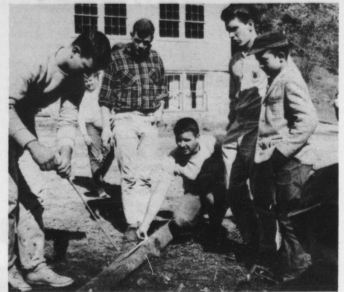
Students work with residents of the Eastern Kentucky area in improving and repairing school buildings. School improvement is one of four major projects of the group.
