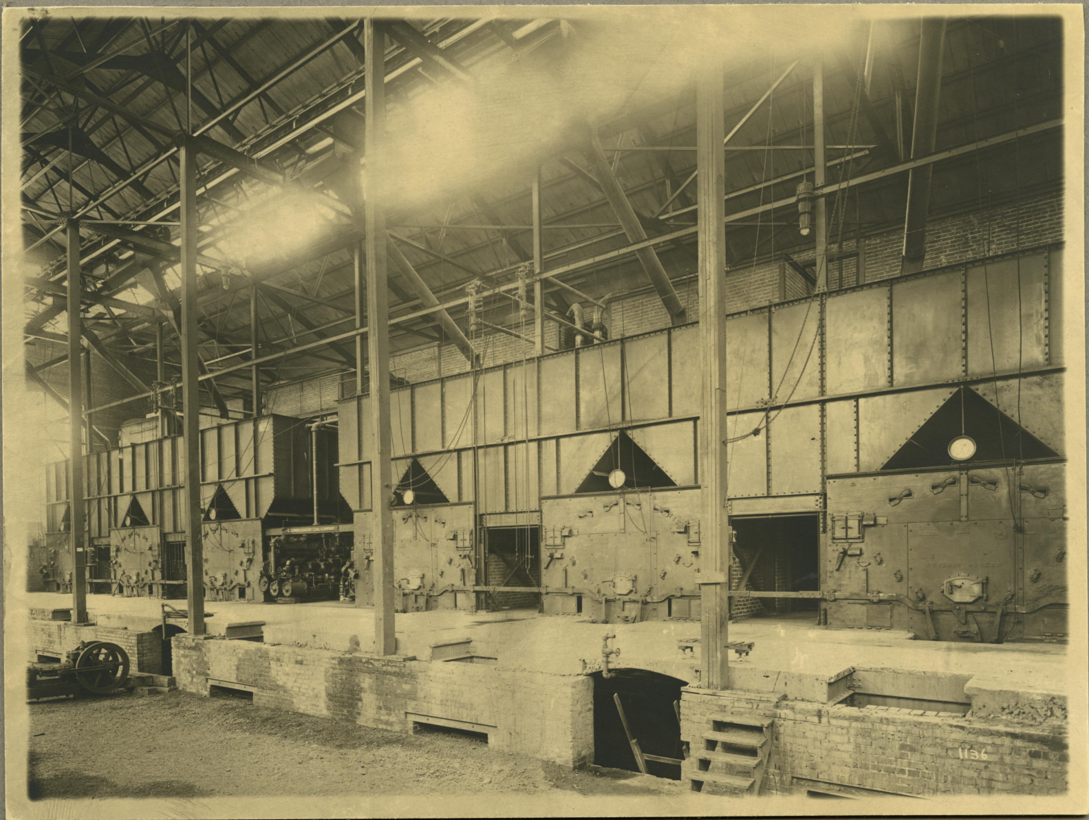
Central Power Plant ~ Boiler Room
