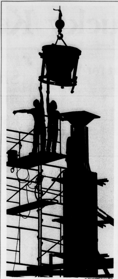
REACHING FOR THE TOP: Construction workers reach for concrete bucket at the Robotics Center yesterday afternoon.
