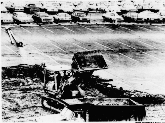
Construction in the parking lot across from the Chemistry/Physics Building has led to the loss of more than 200 parking spaces. UK employees have called for immediate action.
