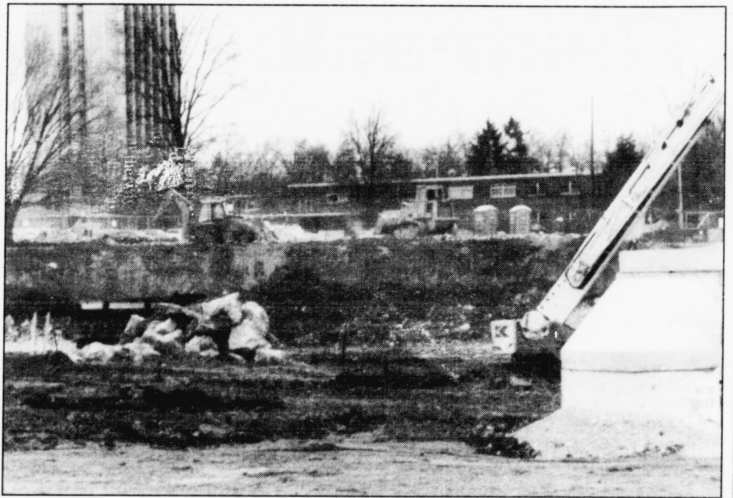
The basement for the new library has been dug, and by the Summer Semester the steel structure will begin to rise above Clifton Park.
