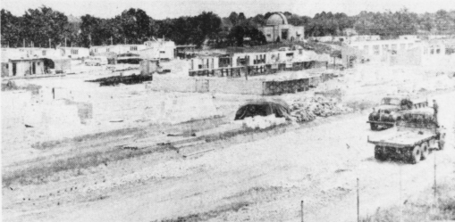
CHRISTMAS GIFT — Work on "fraternity row" is progressing rapidly. The contractor expects to have the six buildings ready by Christmas and the fraternities are scheduled to move in are Sigma Chi, Phi Sigma Kappa, Lambda Chi Alpha, Kappa Sigma, and Pi Kappa Alpha. The sixth building will probably be used as a graduate men's dormitory. —Kernel, July 17.
