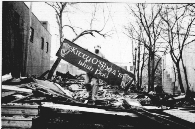
Willie Bodue, a manager at Pazzo's, salvages the main Kitty O'Shea's sign yesterday afternoon after crews demolished the bar.
