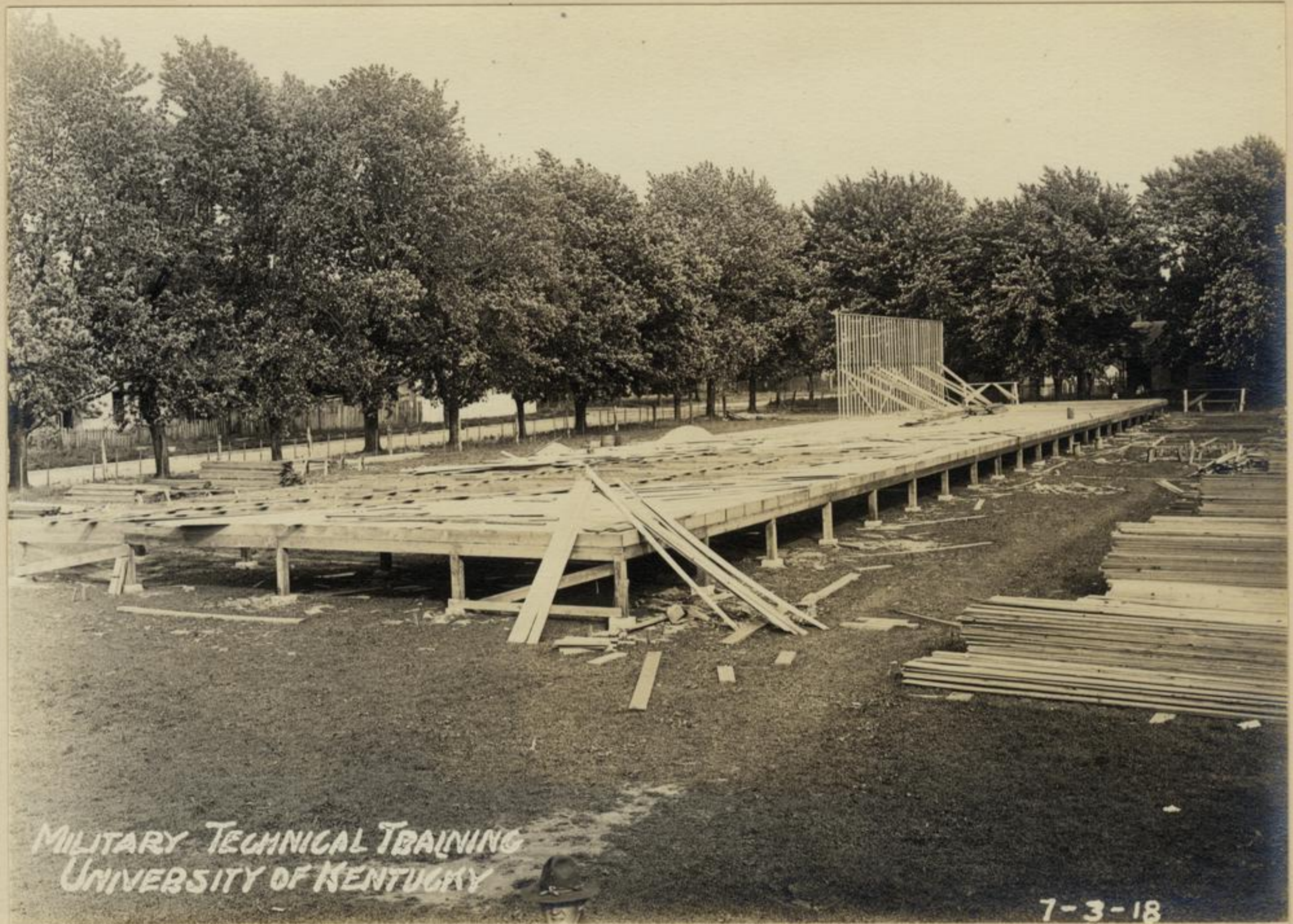
Construction of Barracks by Soldier Mechanics on the Campus University of Kentucky, Lexington, Kentucky
