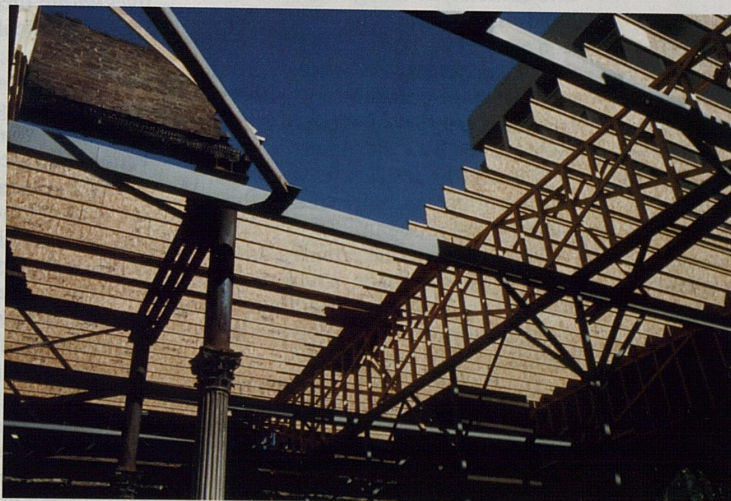
A temporary roof and steel reinforcements are put in place to protect the Administration Building until renovation can begin. The ornate column, one of a pair, survived the fire and will be a part of the building’s redesign.
