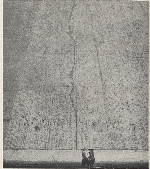
FIGURE 20.—TYPICAL CRACK IN A HEAVILY REINFORCED SECTION.
