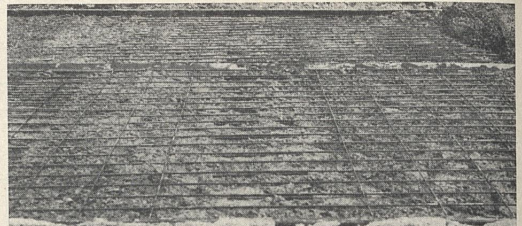
FIGURE 11.—SHEAR DOWEL BARS IN PLACE AT LOCATION WHERE WEAKENED-PLANE JOINT IS TO BE FORMED.
